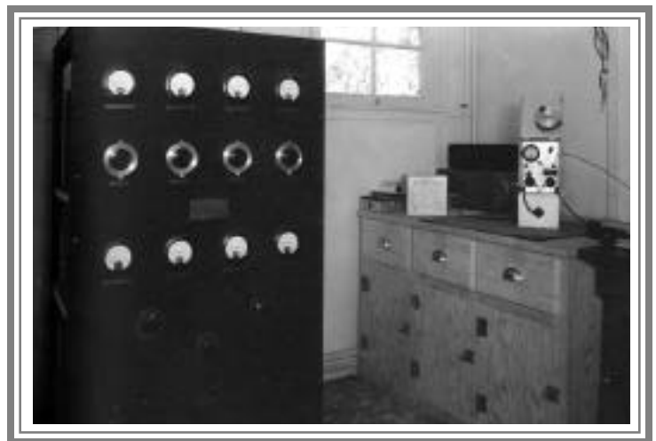
"Radio telephone transmitting station KNDO operating on 2496 K.C. at Park Headquarters. This radio operating room is operated in conjunction with the Electric Shop."
